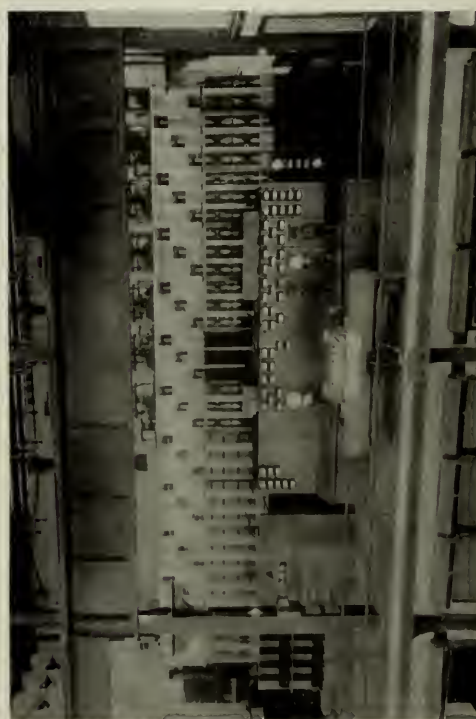
Fig. 9. View of Switchboard Operating Gallery
