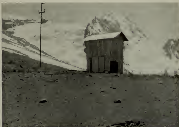
Fig. 7. Lightning Arrester Station at Antaona. Elevation 16,000 ft.
