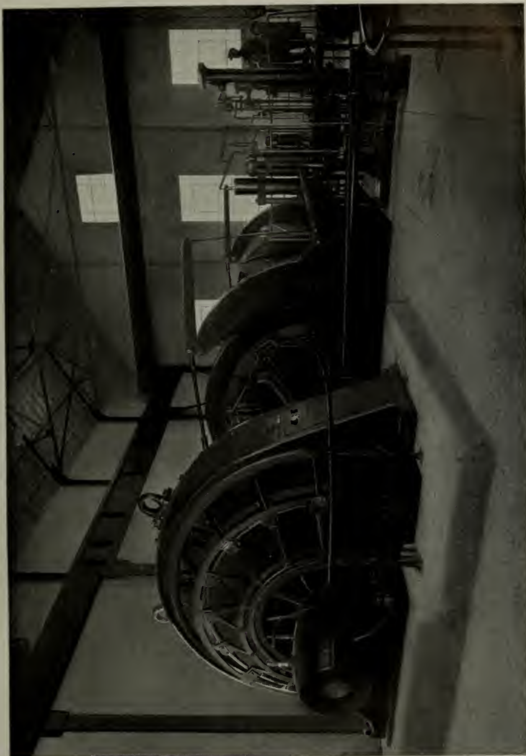
Fig. 1. View of Hoist Motor and Control Equipment
