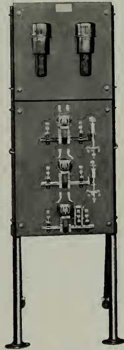
Fig. 7. Time-limit Starting Panel for a Single-phase Motor
