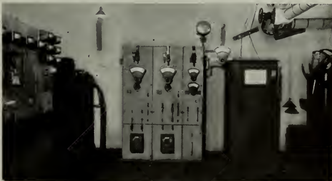
Fig. 6. Direct-current Switchboard in Substation
