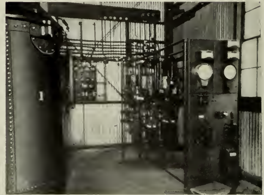
Fig. 3. Feeder Switches and Transformer Room
