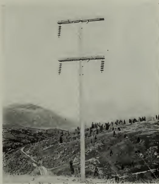
Fig. 4. Standard 100,000-Volt Wood Pole Transmission
