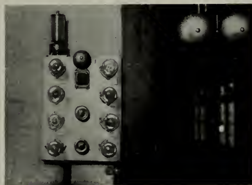
Fig. 27. Improvised Combination Bell and Light Indicator to Show High or Low Water Levels in Tanks or Flumes
