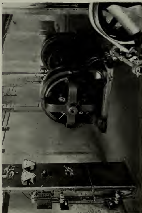
Fig. 20. Motor-generator Set for Operating Variable Speed end of Paper Machine
