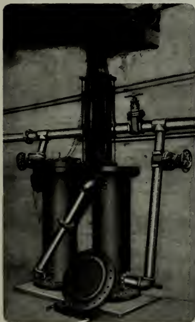
Fig. 12. Electric Air Heater for Hoist
