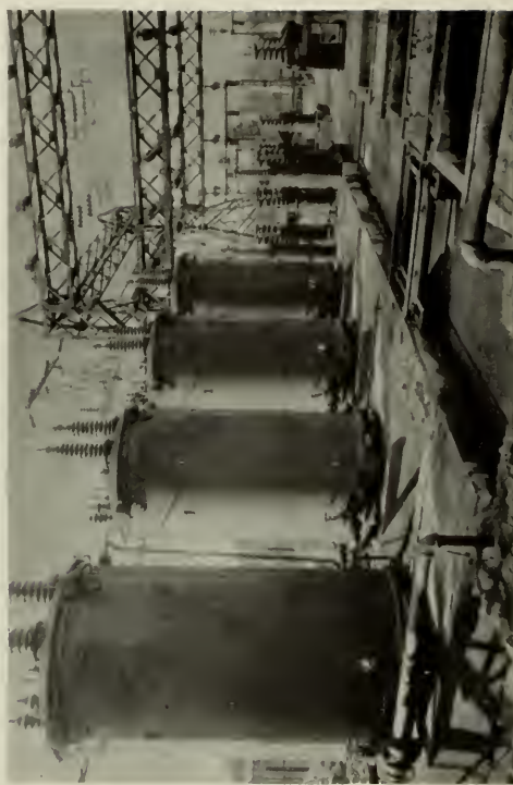
Fig. 17. View of Typical Outdoor Substation
